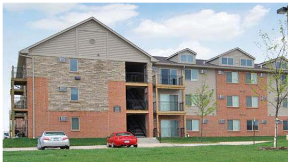
Inappropriate application of stone over brick
